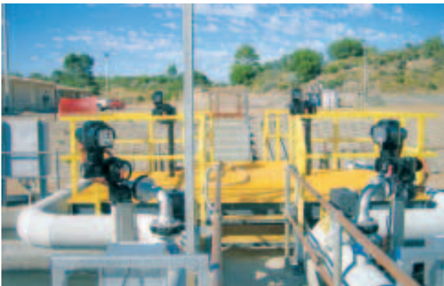
Multi-turn actuator/worm gearbox combination in a water treatment plant in Australia.
