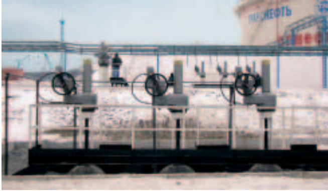
AUMA multi-turn actuators SA in combination with spur gearboxes in Siberia.
