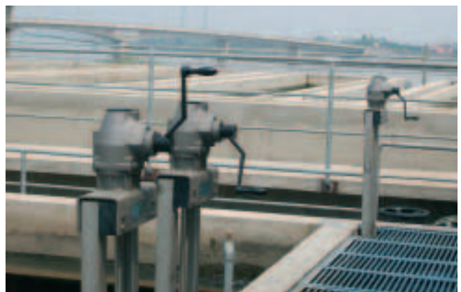
Bevel gearbox for manual valve operation in a Vietnamese sewage plant
